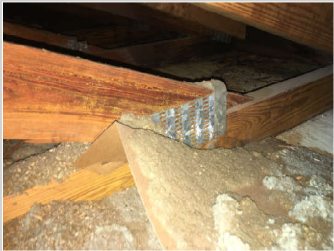
Toe Nail - Not Meeting Nail Requirements
