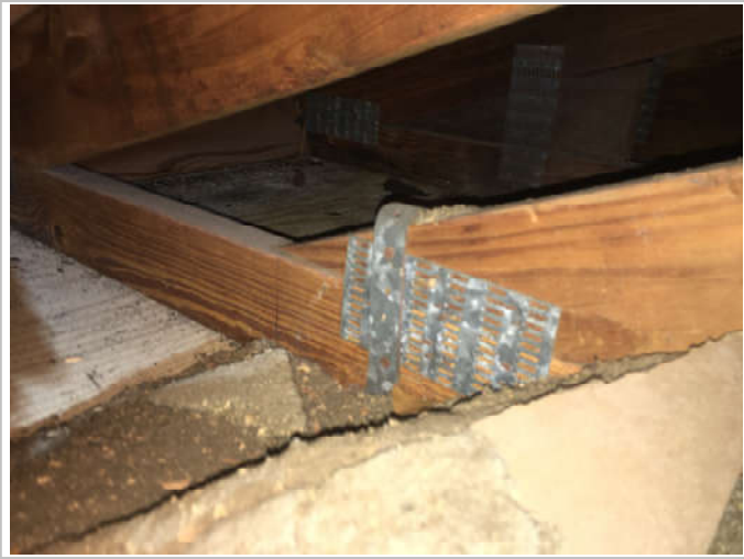
Toe Nail - Not Meeting Nail Requirements
